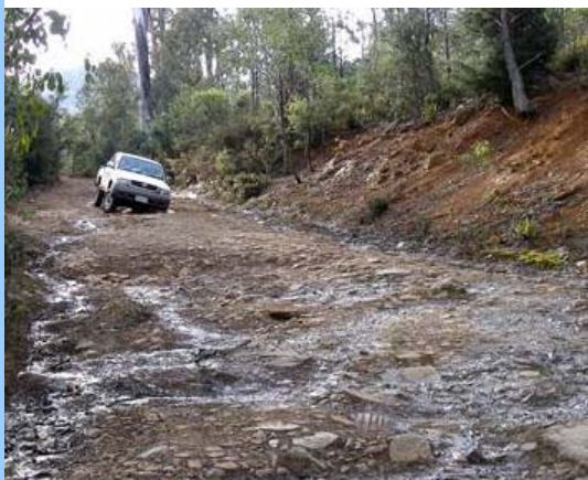
The road into Woods Lake before the works: 4WD track at best and not for those wanting a comfortable ride.
