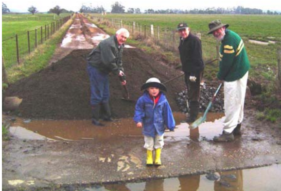
Ted Whinnett, Tony Ritchie, Ivan Iles and Innes Ferrier hard at work preparing Fischeies Lane for early season traffic
